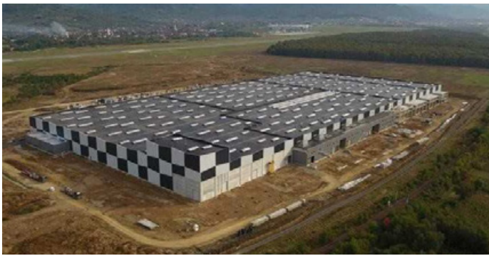
The new Montana Aerospace plant in Baia Mare, Romania, after its completion in spring 2021 and coping with the COVID-19 crisis, with a production area of more than 80,000 m 2 , is to create many jobs and implement attractive orders.
